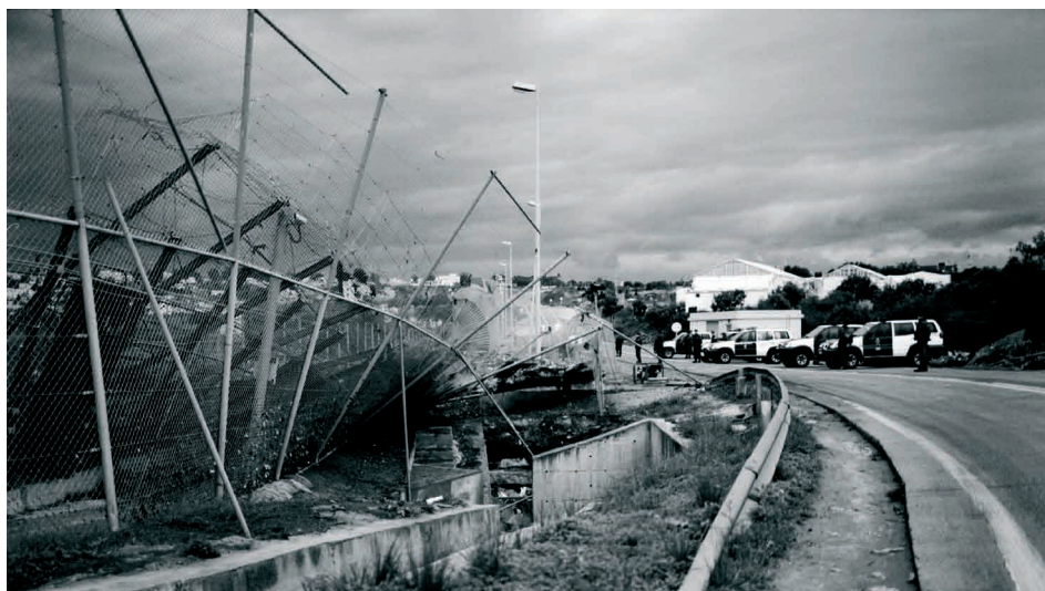
La valla-November 2008, heavy rain has destroyed groundwork of the fence, Melilla Spain, 2008
